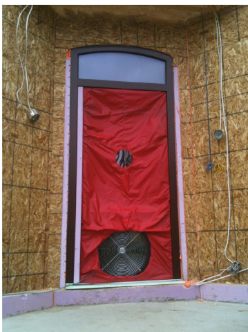
Front door replaced with equipment to test air leakage at the Hoyer house. Increased air pressure is developed inside the house by the fan, and the rate of air leakage determined.
